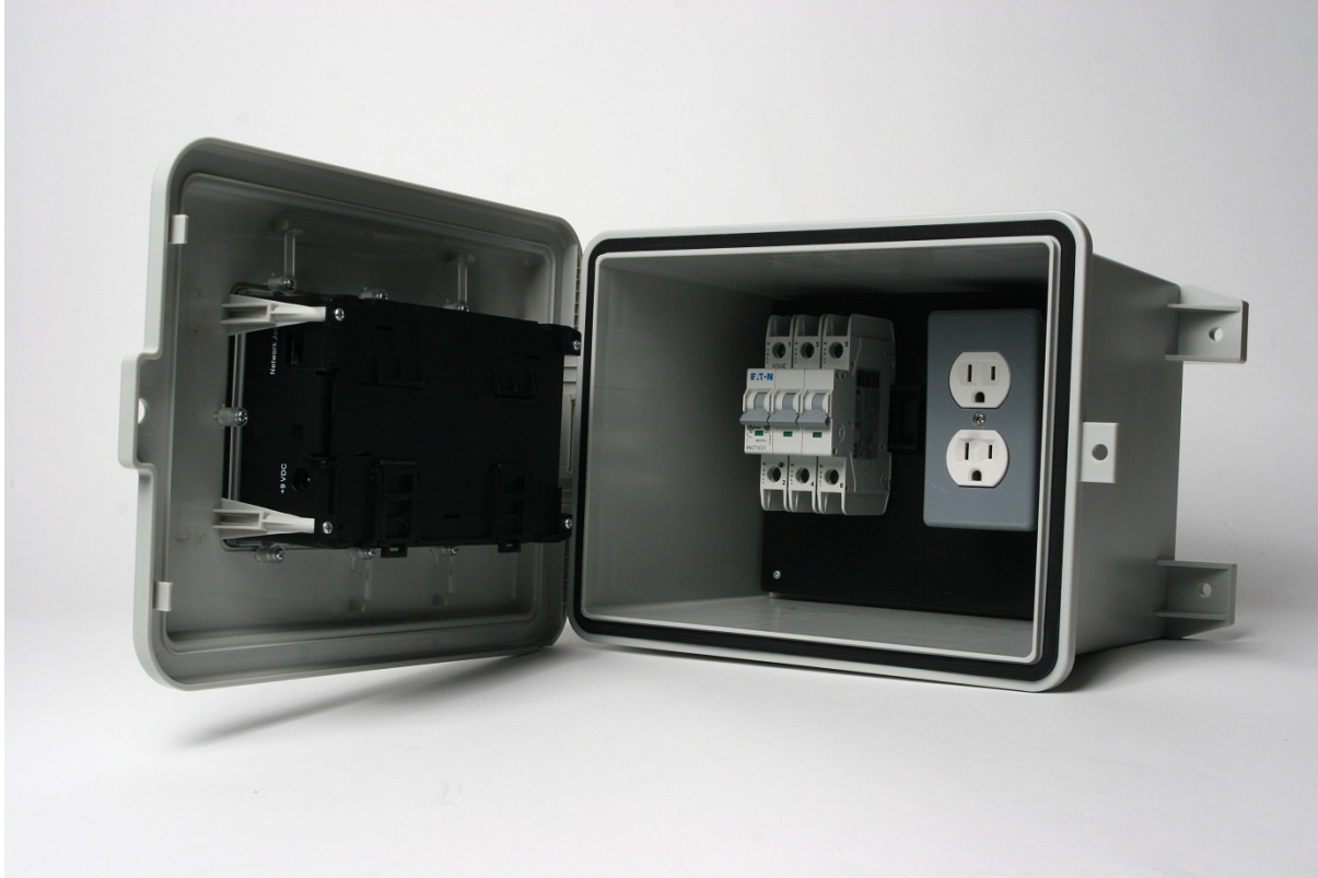
Figure 2: Note the separation between the breaker block and the Ethernet port on the meter.
